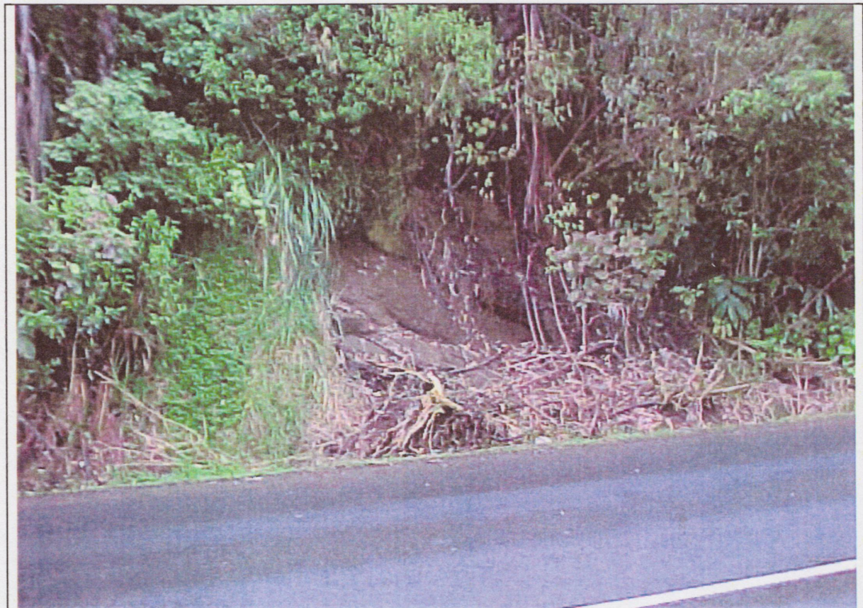
The northern side of Waima Road near Nihotupu Filter Station – showing exposed sandstone
