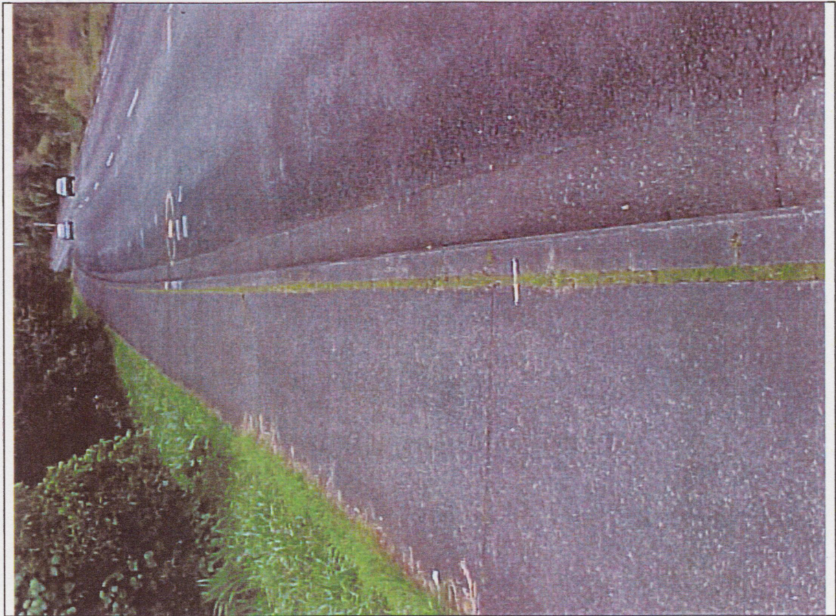
Looking West along Waima Road – showing minor sideling fill movement
